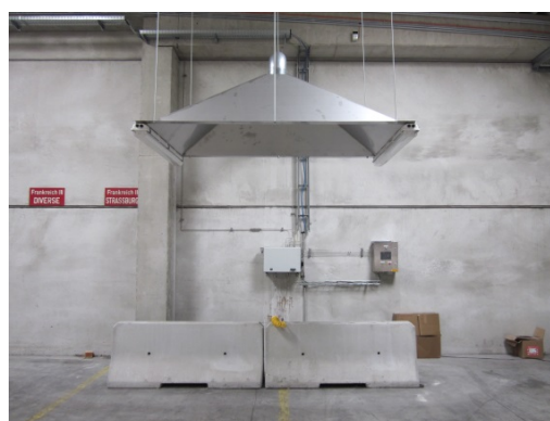
Figure 4: Indoor hydrogen refuelling station
